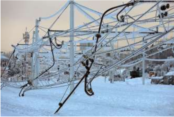
Damage from freezing rain. Credit: Wikipedia.
